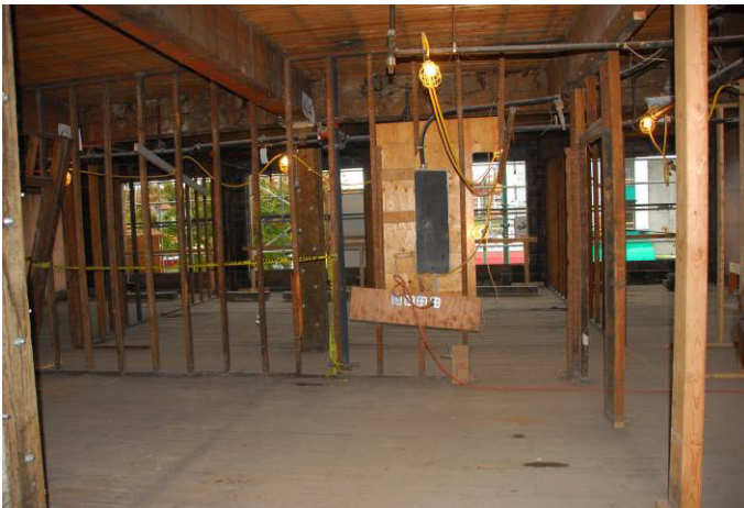
An overview shot from one of the upper floors shows the extent the building had to be gutted.
