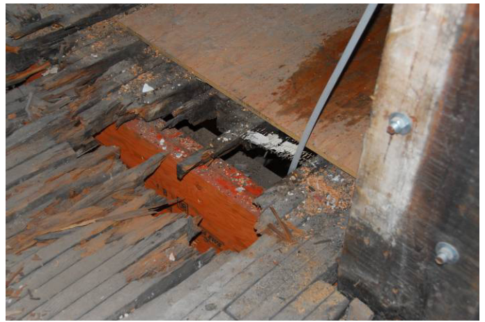
A rotten floor now supported by a new beam (orange) below.
