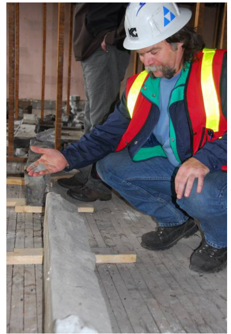
Project Superintendent Ron Gust easily removes portions of the stone windowsills and crumbles it in his hand.
